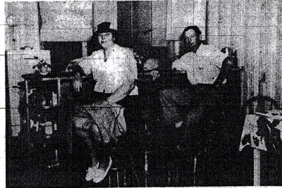
Top picture shows the foundation of another new cottage. Mr. and Mrs. J. D. Dance, of Richmond are the builders. Mr. Dance and sons are working while Mrs. Dance and a neighbor, Mrs. Lovelace, look on. Next picture shows the corner of Bayshore Drive and Evelyn Ave., looking down Bayshore Drive. Left to right; completed cottages of Mr. and Mrs. Ben Weeks, of South Richmond and Mr. and Mrs. Hardy Weeks, of Petersburg Pike, and the partially completed cottage of Mr. and Mrs. Cary Lovelace, Petersburg Pike. Next View from the beach, showing, left to right, completed cottage of Mr. and Mrs. W. L. Petway, McGuire Park, Richmond, finished in five days; nearly completed cottage of Mr. and Mrs. John E. Seaton, Sandston, and partially completed cottage of Mr. and Mrs. Lucius S. Walker, Petersburg Pike. House at rear is that of Mr. and Mrs. Lovelace. Lower picture shows Mr. and Mrs. Petway, seated at the snack bar in their completed cottage facing the beach. They were just going fishing when they stopped to pose for a Gazette-Journal protographer.
